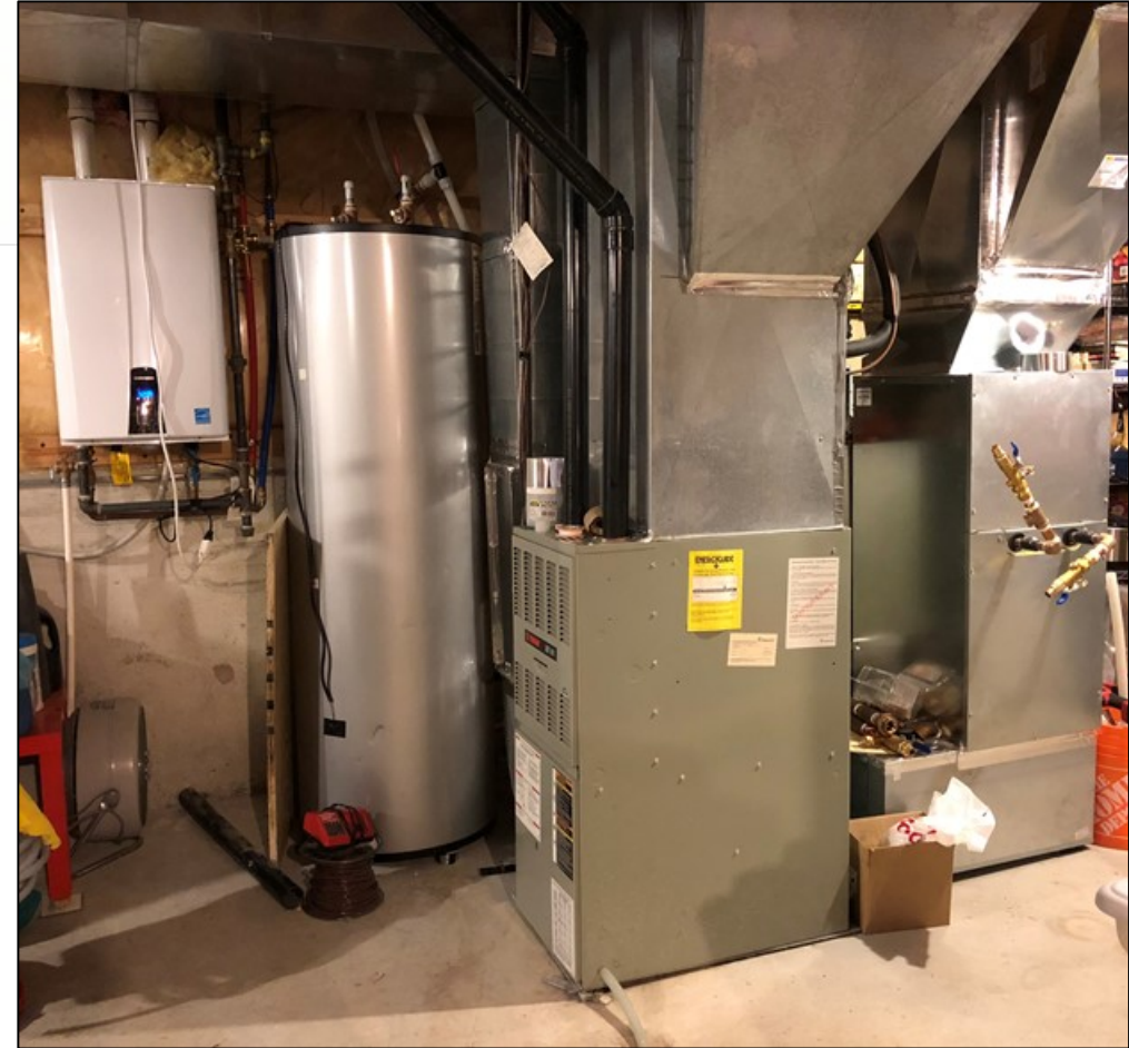
THP water heater
