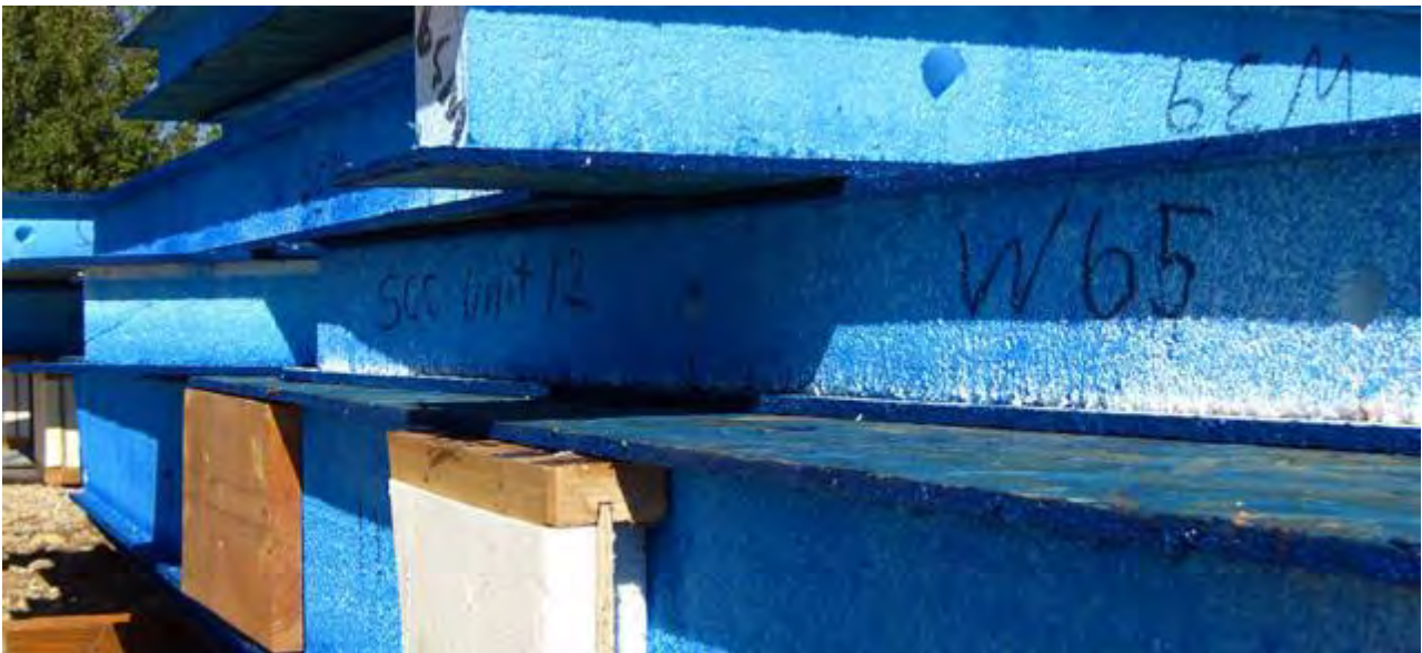
Figure 5: 6" wall and 12" roof Structural Insulated Panels for the Snow Creek Project on-site in Park City, Utah, 2011
