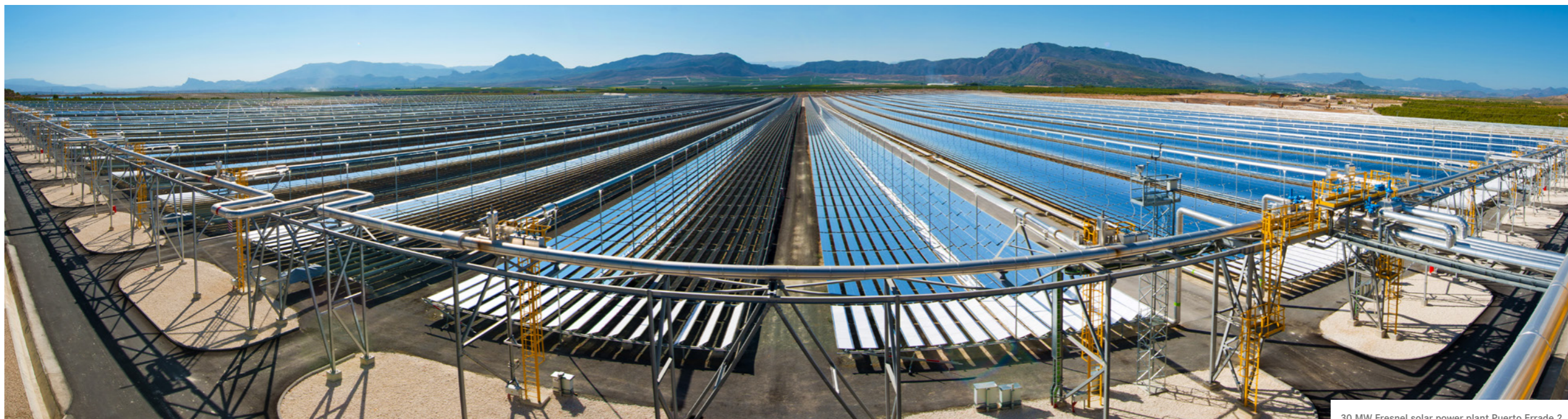
30 MW Fresnel solar power plant Puerto Errade 2, Calasparra, Spain (FRENELL GMBH)
