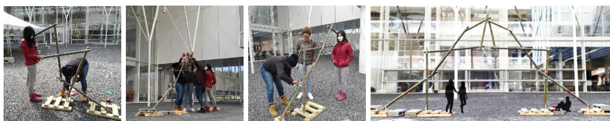
Figure 10. Installation (from left to right): setting pedestal, linking up 4-bar pin connection, setting translatable pin connection, and final configuration
