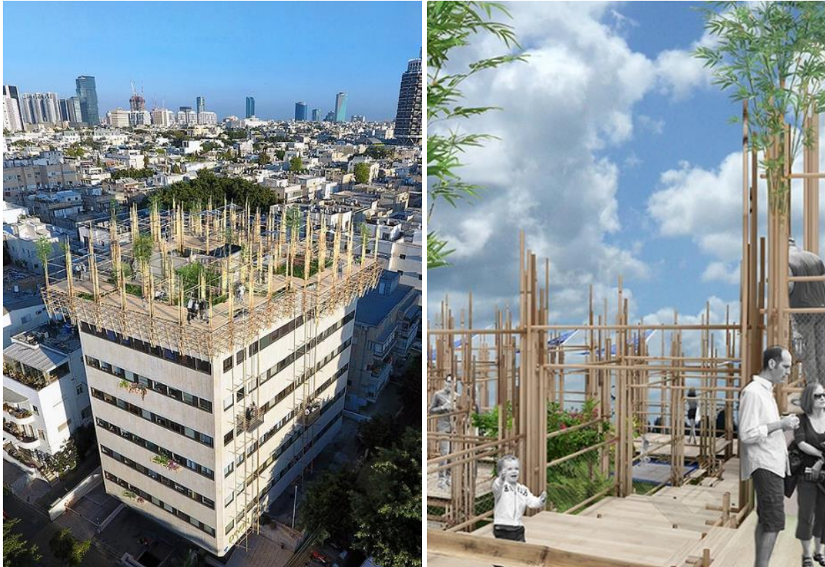
Figure 3. Example of bamboo scaffolding construction on rooftop of existing building to create new public areas.
