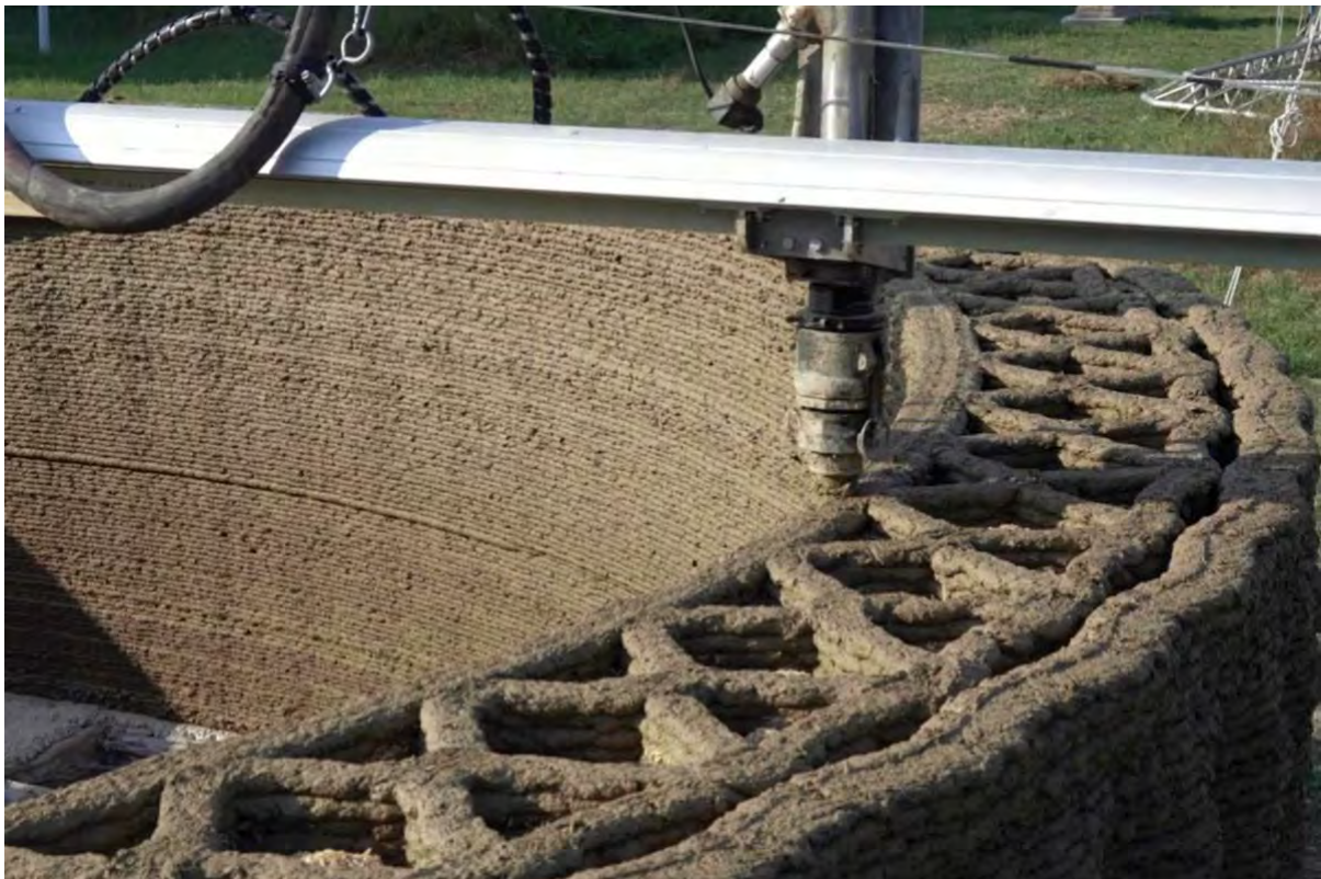
Figure 28. A moment in the construction of 'Gaia' prototype developed and built by the Italian company WASP s.r.l.
