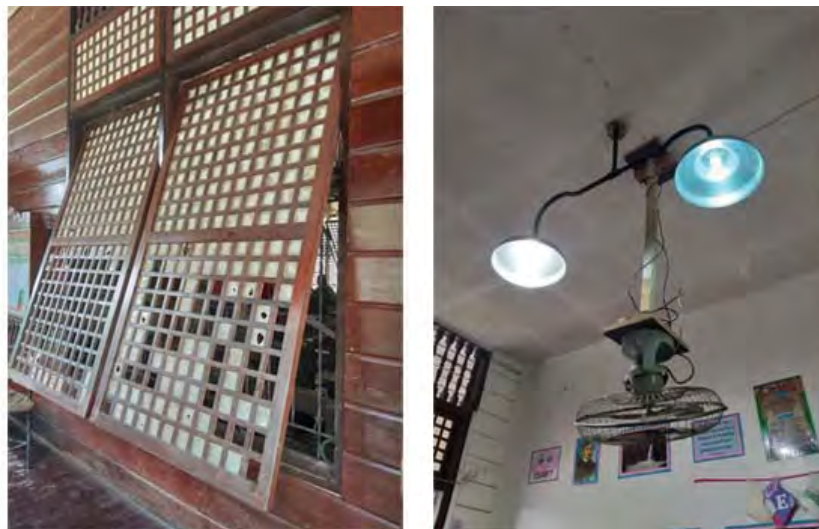
Figure 43. Typical features, left to right: (a) Capiz window open 20 degrees, (b) aluminum reflector with compact fluorescent lamp (CFL)
