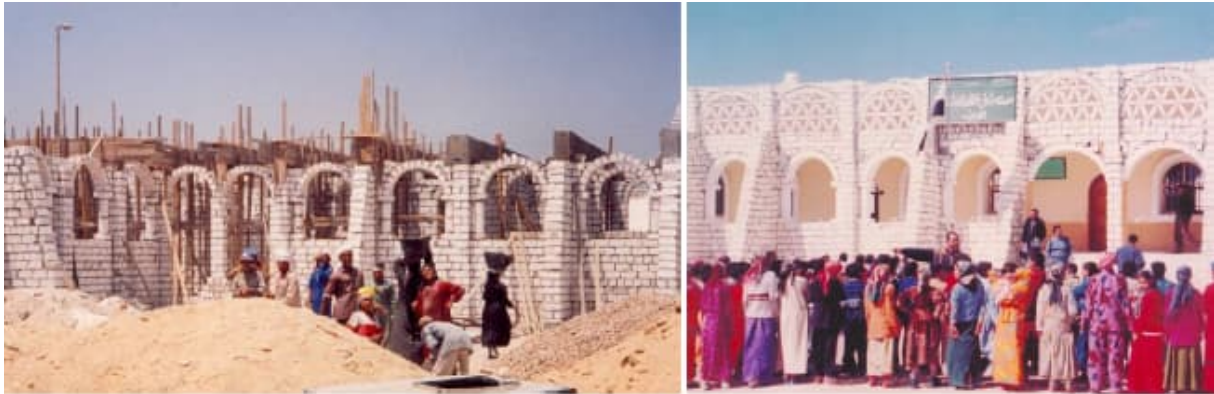
Figure 8. Pictures showing construction works (left) and first day of school after completion (Right)
