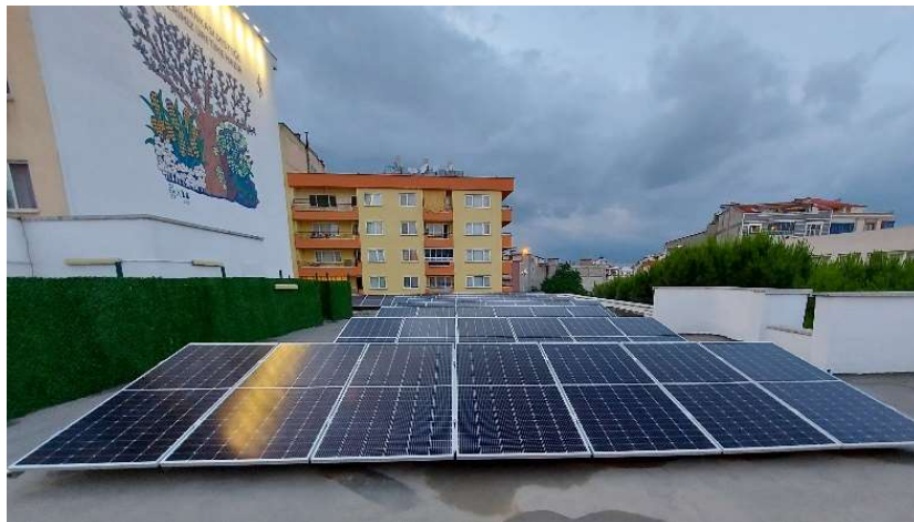
Figure 10. Roof solar panels
