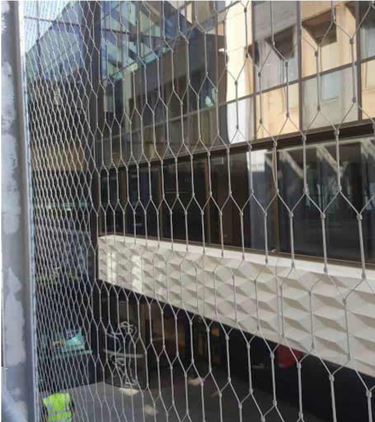
Figure 13. Photograph of built outcome for university library balcony showing full height decorative balustrade mesh detail.
