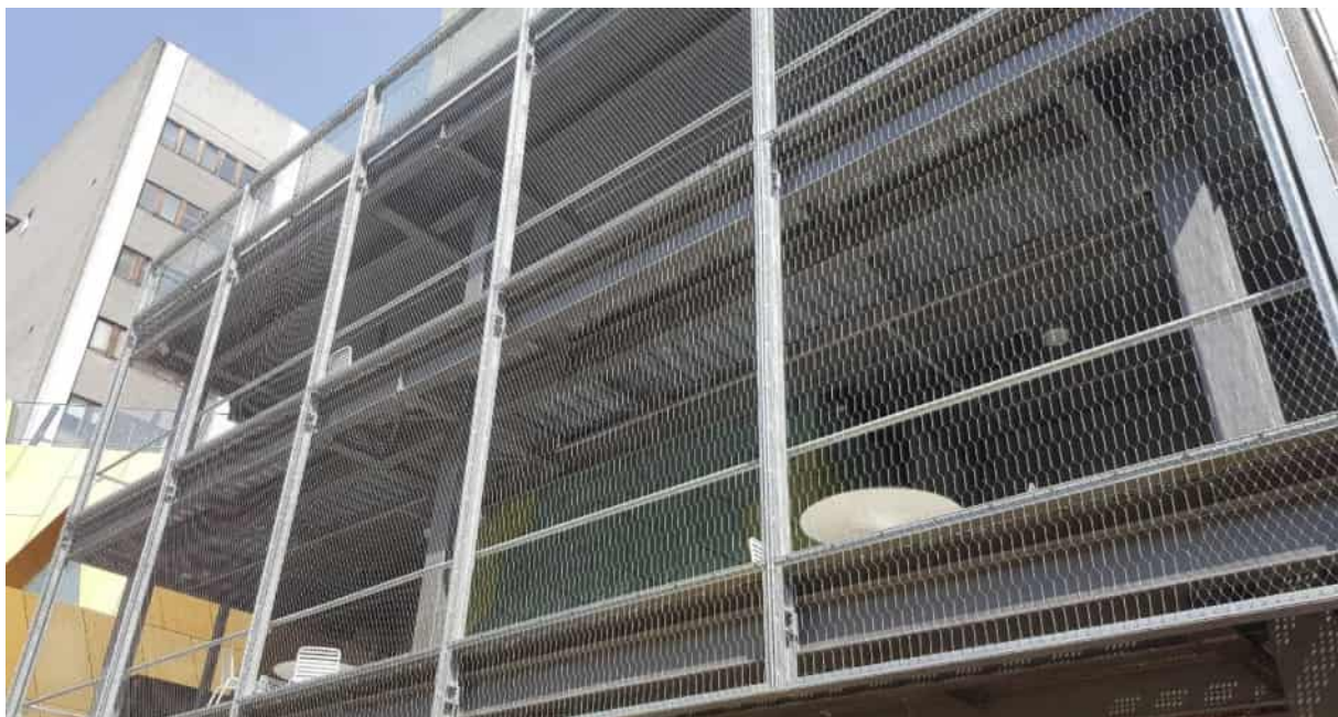
Figure 12. Photograph of built outcome for university library balcony showing full height decorative balustrade mesh detail.
