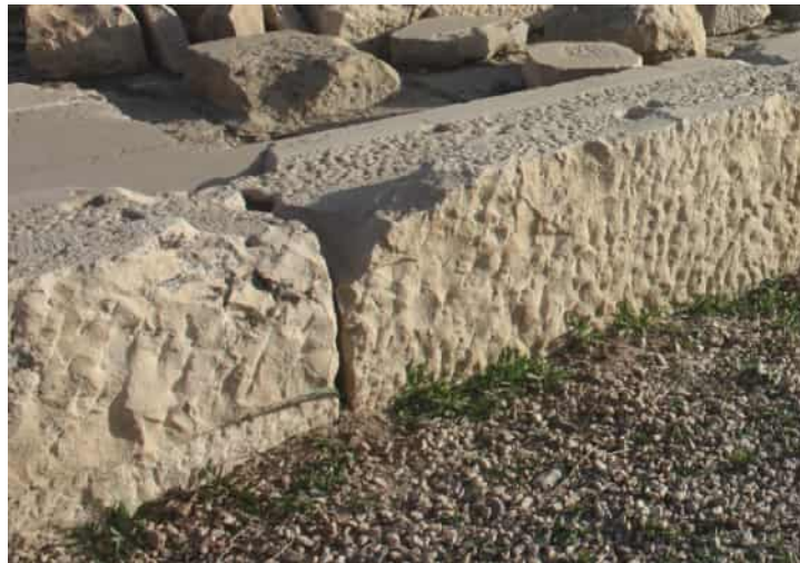
Figure 2. Example of degraded masonries in need of pointing with compatible mortars (Pasargadae, Iran)
