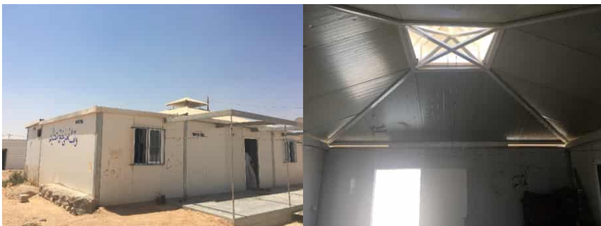
Figure 4: One man dismantled one of his caravans to build a new roof between the other two caravans, creating a living space with a ventilated roof to overcome the summer heat.
