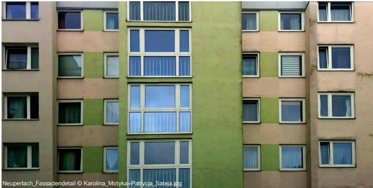
Figure 3. Decaying building substances of Neuperlach
