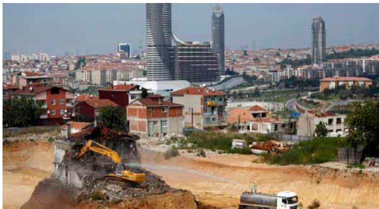
Figure 12. The process of demolition of the last remaining gecekondulı in Fikirtepe [URL 2]
