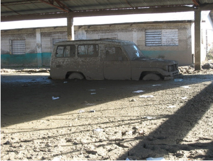
One section of the schoolyard. Note the high water mark just under the eaves.
