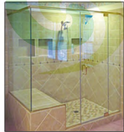
Greater chance of leakage
