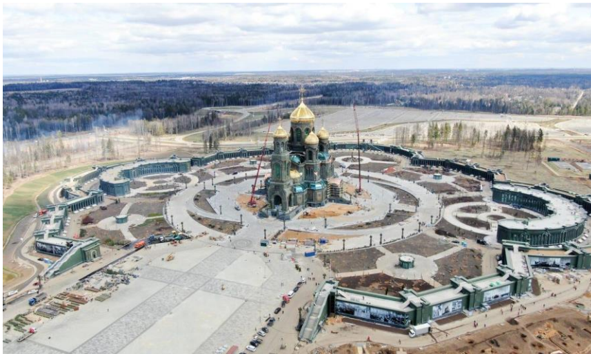
An aerial view of a military cathedral during construction works in April 2020. Denis Voronin/Moscow News Agency/Handout via https://www.businessinsider.com/russias-massive-cathedral-rumored-made-
