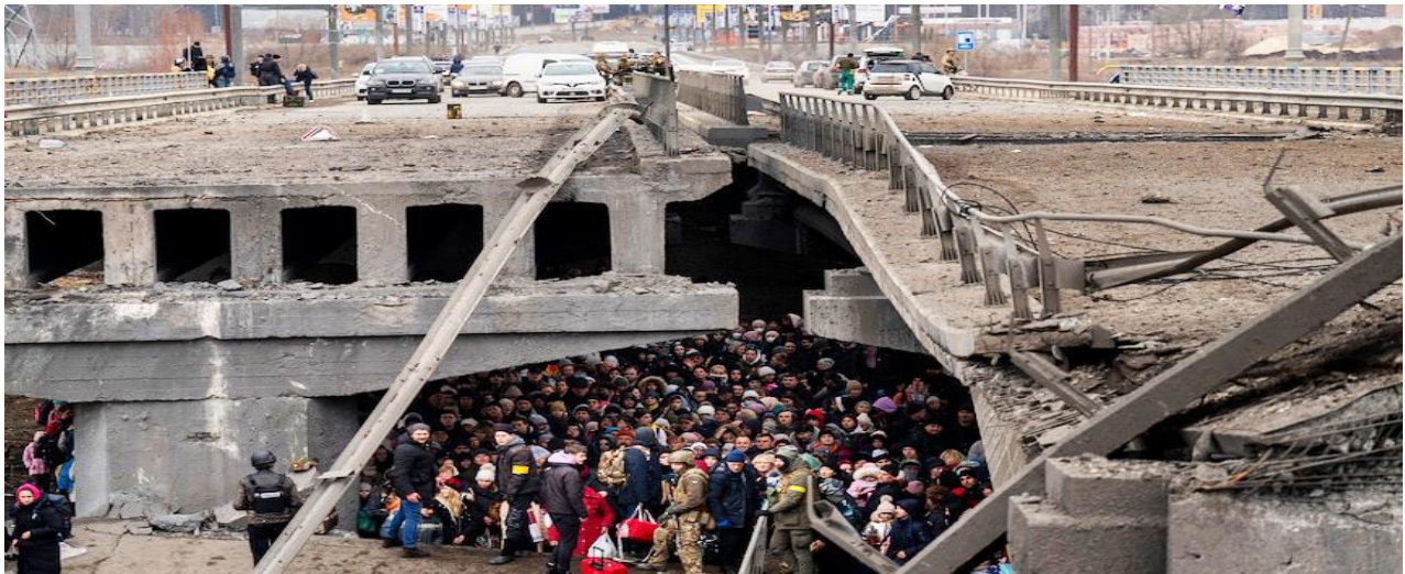
The bridge over the Irpin River, near Kyiv, destroyed by a Russian air strike. Photo Credit: AP: Emilio Morenatti
