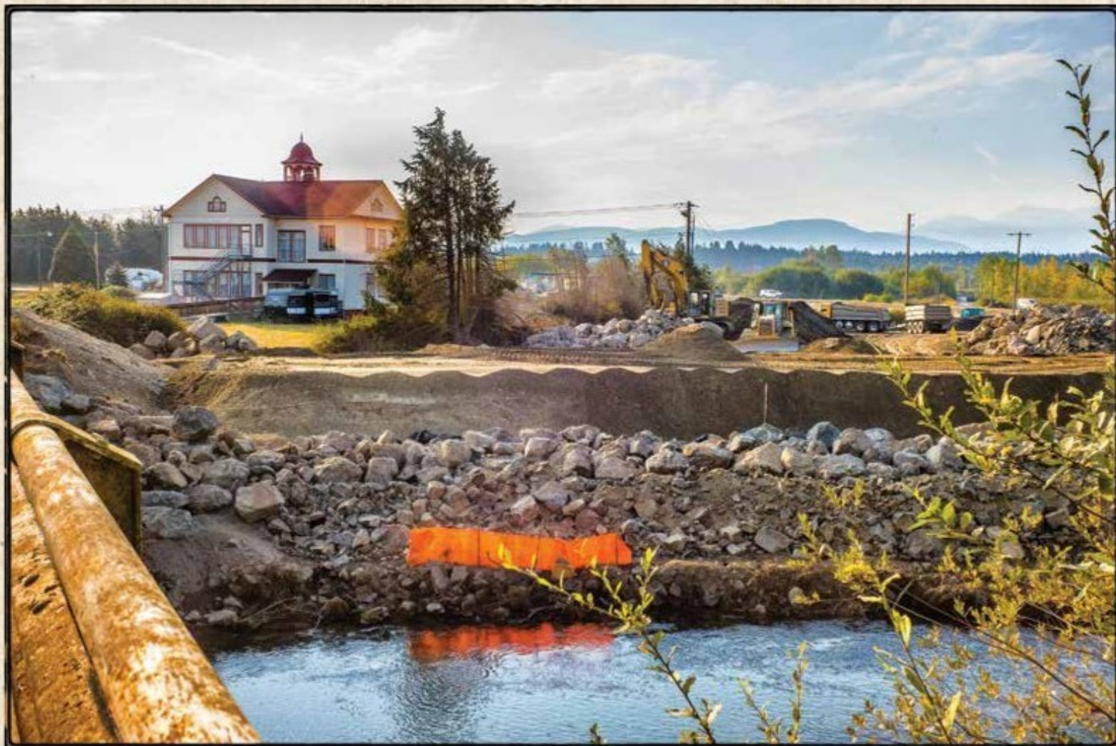
New Levee being constructed near the historic Old Schoolhouse. Photo by Bob Lampert
