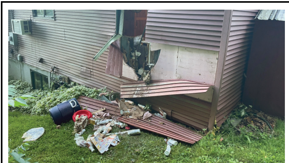
Damage to a building exterior caused by a bear that became habituated to a birdfeeder on the property. ~ VTF&W photo
