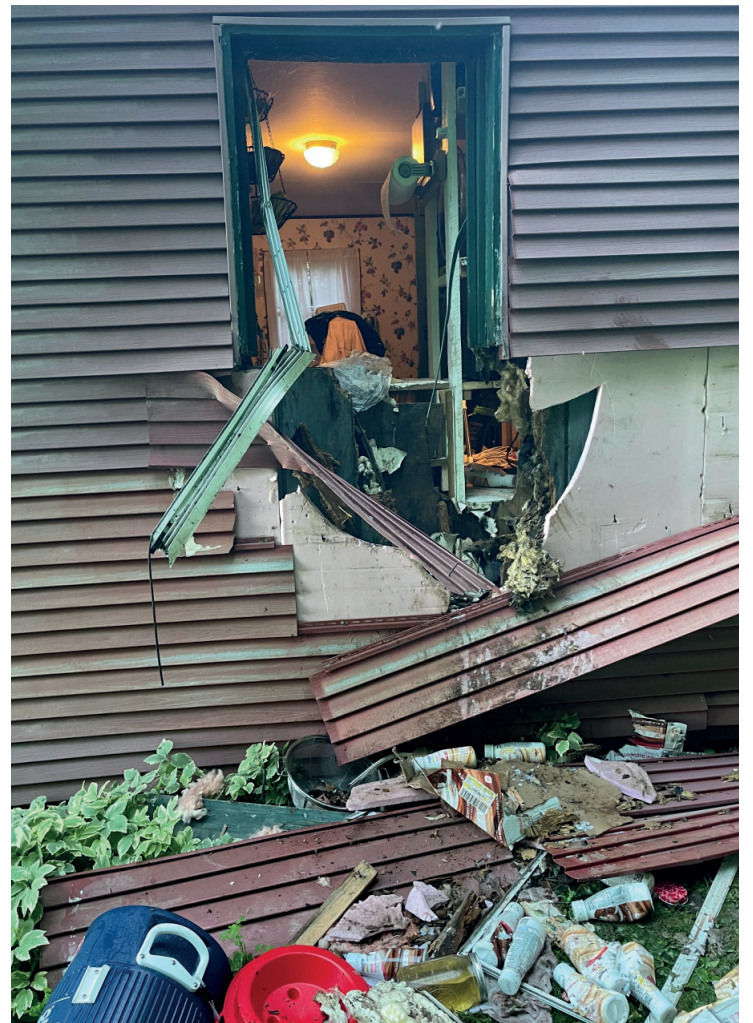
Building damage caused by a bear that had become comfortable around a Vermont residence and attempted to access the kitchen in the summer of 2022.
