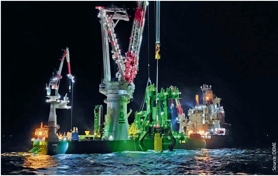
The installation vessel Orion recently completed installation of the largest-ever monopiles at the Arcadis Ost 1 wind farm
